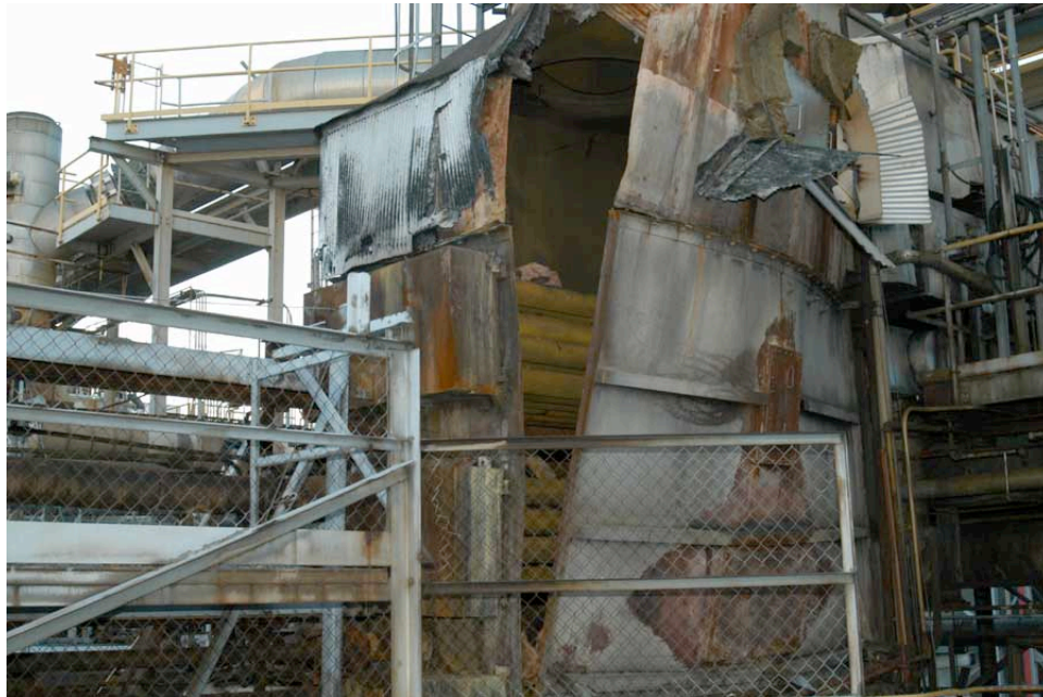
Figure 2: Ruptured Convection Section
